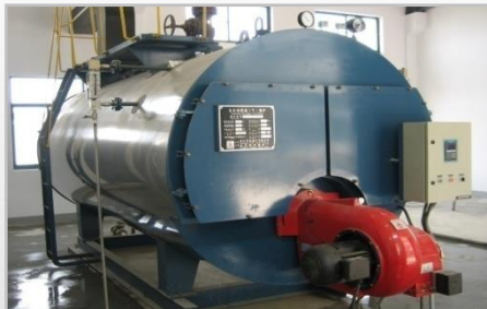
Steam Boiler 蒸汽锅炉
